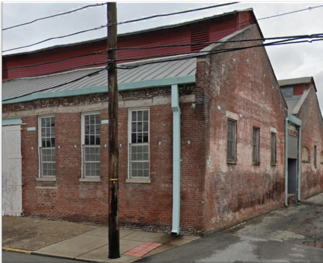
Plate 7: Looking toward the south and rear elevation of the Louisville Streetcar Barn
